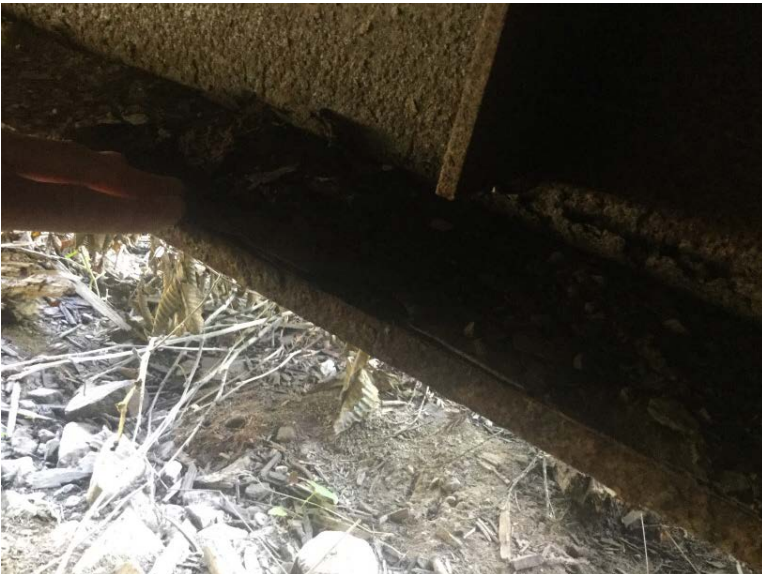
Town jump span - corrosion on girders
