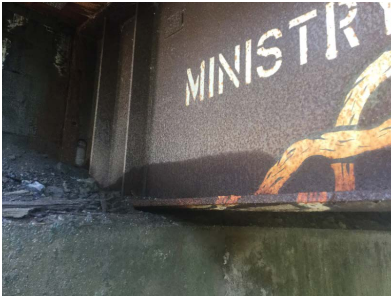
Town side jump span - dirt on girders
