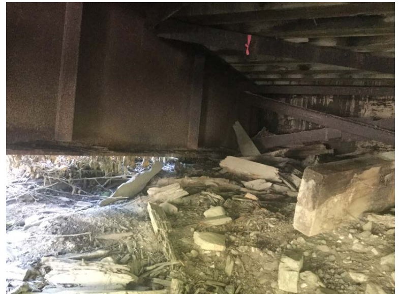
Town jump span - corrosion on girders
